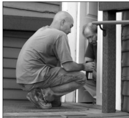
Garrett Irwin and Noah Bradley confer on water damage during Ellwood’s restoration. Visitors get a sneak peek at the work on February 14th.
